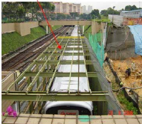
Erection of protective steel portal frames over MRT tracks with steel plates for lifting operations close to RTS tracks
