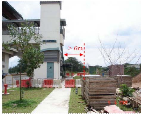
Storage of combustible materials outside 1 st reserve
