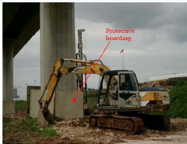
Steel hoarding erected around RTS viaduct column for operation mechanical equipment beside column
